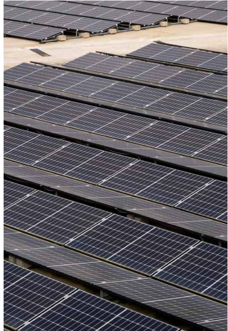
Photovoltaic panels on Wevelgem (B) site
