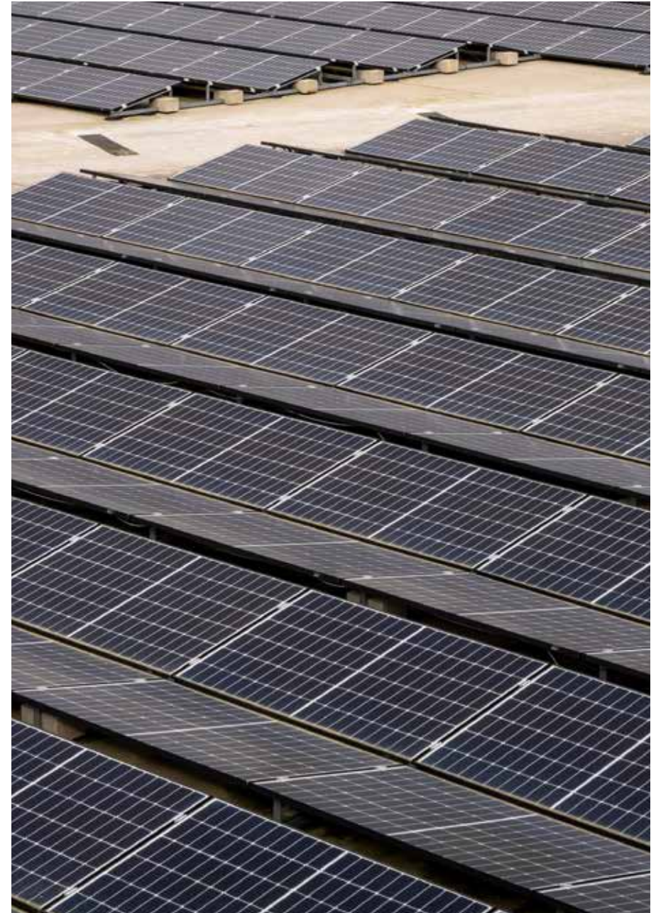
Photovoltaic panels on Wevelgem (B) site
