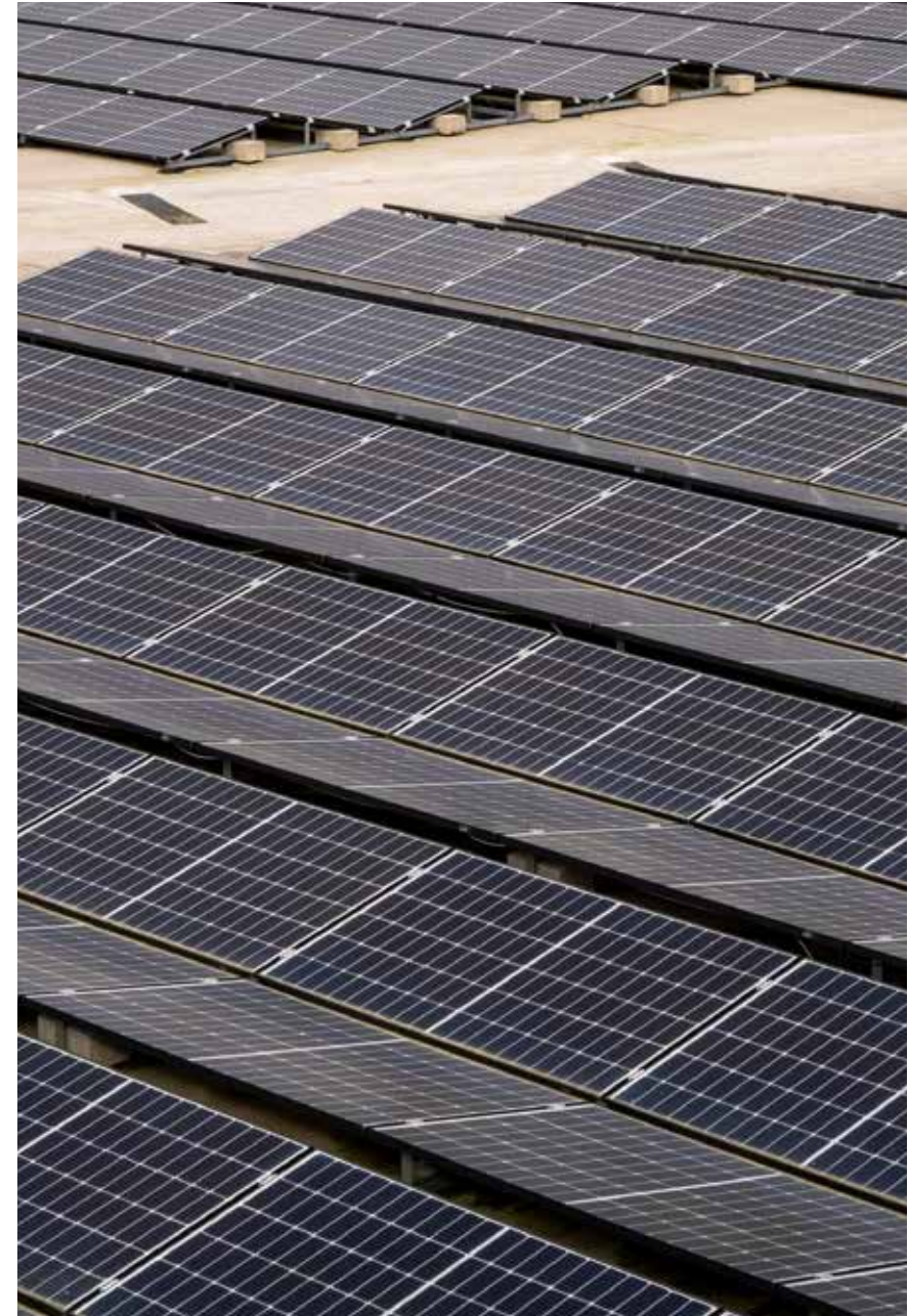
Photovoltaic panels on Wevelgem (B) site
